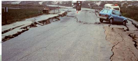
Fig. 10 Earthquake of Loma Prieta - California (1989). Source: https://goo.gl/phfGFU
